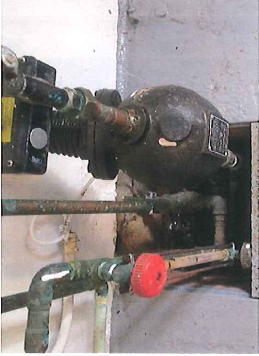
Pumphouse Lower Level – Low Level Cutoff (Photo No. 4477)
