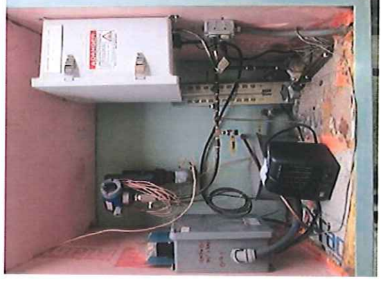
Storage Tank Control Panel (Photo No. 4444)
