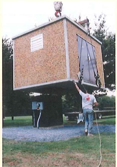
Transformer Substation (Pre-assembled building delivered with hole in floor to fit over transformer)
