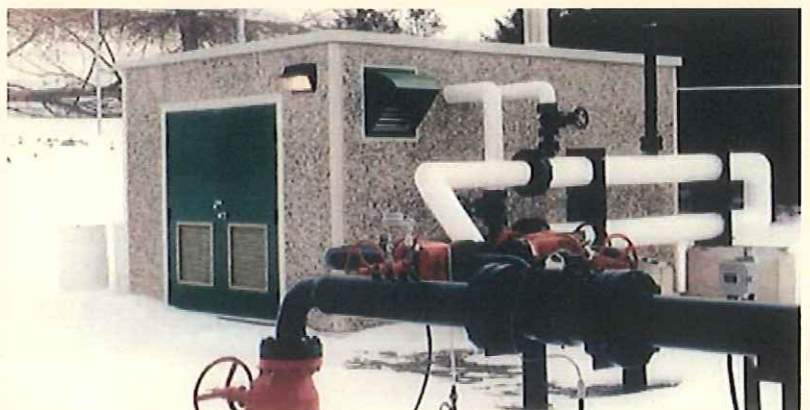
Pump Enclosure, Ontario, Canada
