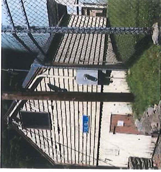
14' x 10' Pumphouse (Photo No. 132127)
