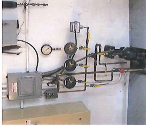
Pumphouse Lower Level - Booster Pump Controls/Gauges (Photo No. 4475)
