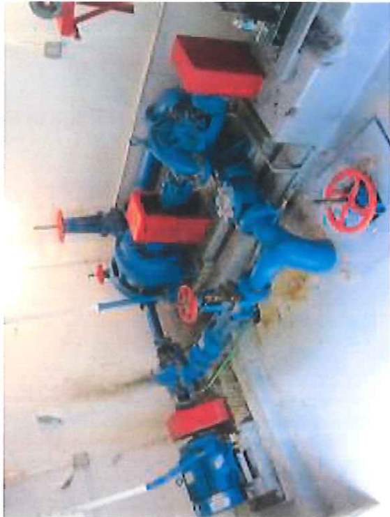
Pumphouse Lower Level – Booster Pumps (Photo No. 4502)
