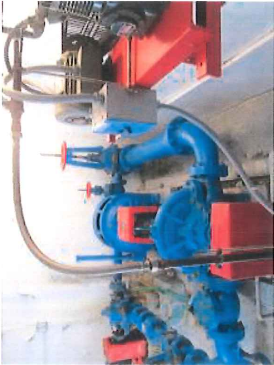
Pumphouse Lower Level – Booster Pumps (Photo No. 4492)
