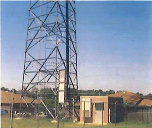
Communications Equipment Housing, Chicago, IL
