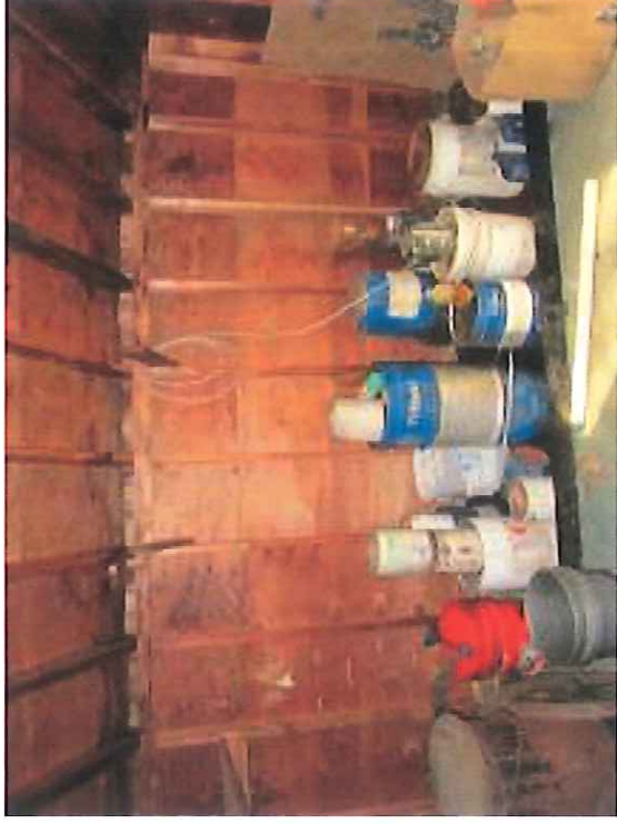
Pumphouse Upper Level – Chemical Storage Area (Photo No. 4454)
