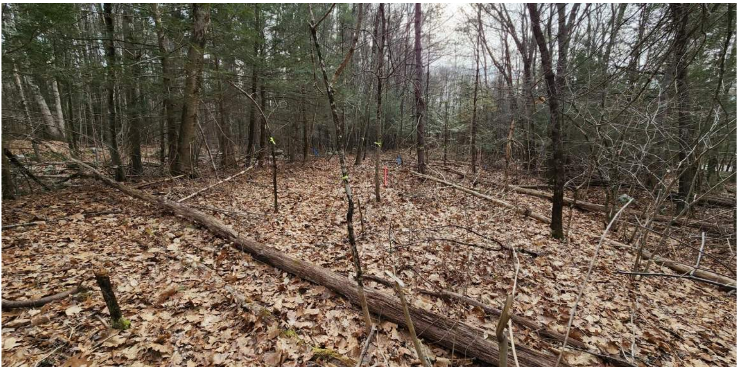
Photo #6: Overview of historically used, abandoned portion of Podunk Road. Soil Borings B-2 is visible in the foreground. An existing culvert is indicated by stakes with blue flagging. Facing west.
