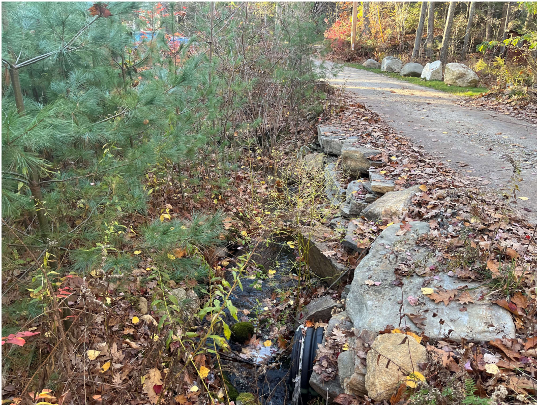
Photo 8 taken by EBT, Inc. on 10/29/2022 – Showing the repair & replace of the ~18’ of historic stone wall which holds the road in place and was missing capstones.
