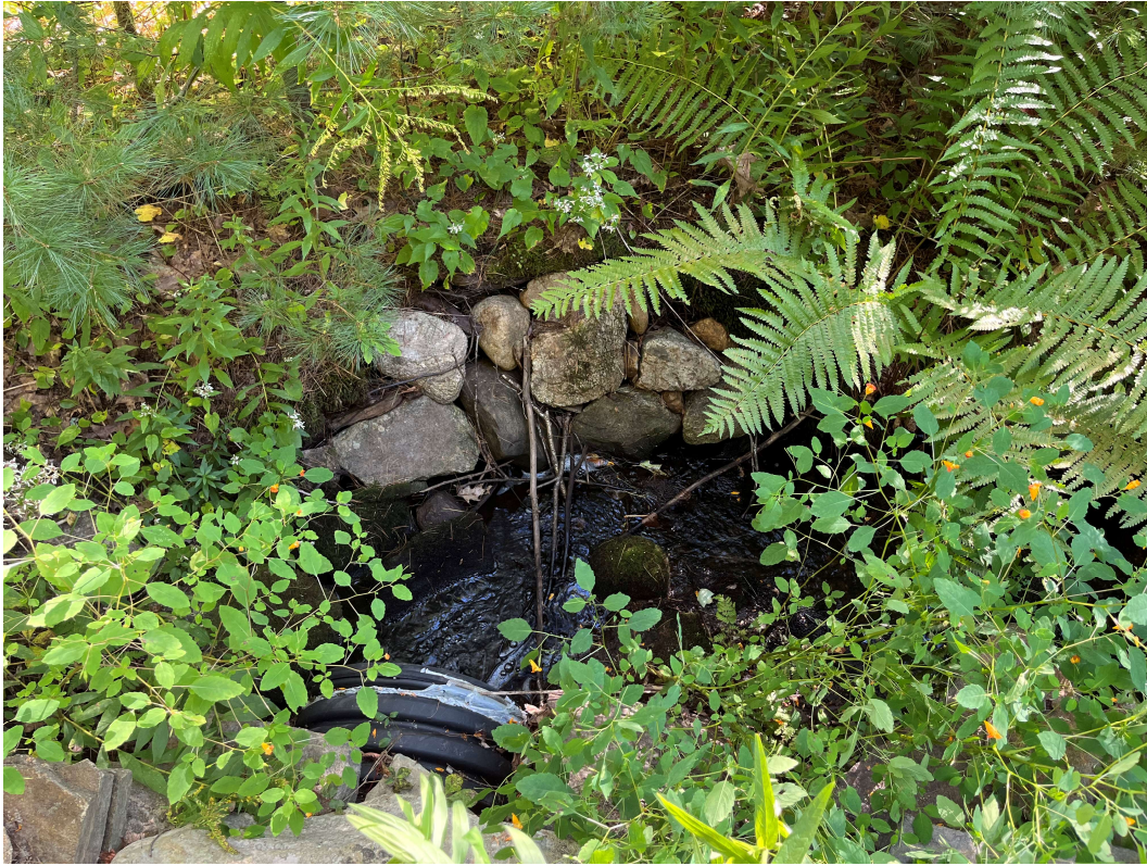
Photo 6 taken by EBT, Inc. on 9/17/2023 – Showing the 10”-12” diameter boulders in the undercut area within the perennial stream at the outflow of the Leadmine Road culvert directly east of the house to stabilize the bank.
