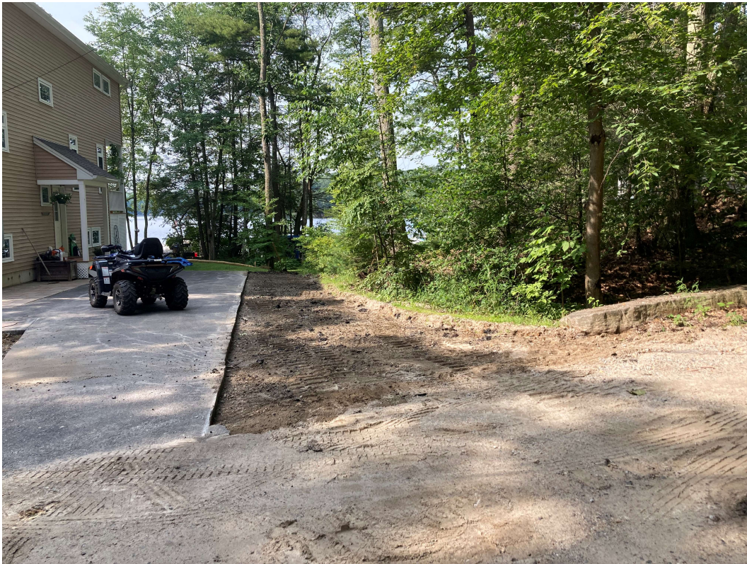
Photo 4 taken by EBT, Inc. on 8/7/2021 – Showing the 498.7 square feet of asphalt was removed and replaced with ¾” crushed stone.
