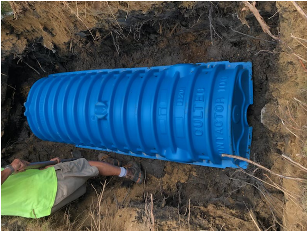
Photo 5 taken by EBT, Inc. on 9/7/2021 – Showing the installation of the C-100HD Cultec unit on the southwest corner of the house which receives roof runoff.
