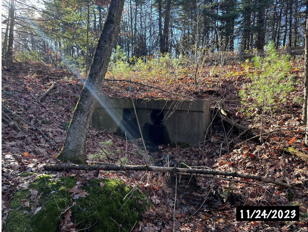
Picture 2. Headwall and double RCP. Haynes St. immediately behind headwall. Blue flag numbered WF-33 can be seen near the center of the headwall.
