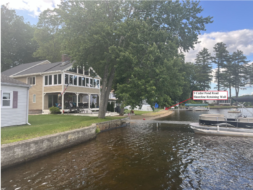
Photo 2 taken by EBT, Inc. on 6/21/2023 – Showing shoreline retaining wall/edge of resource area (in background).
