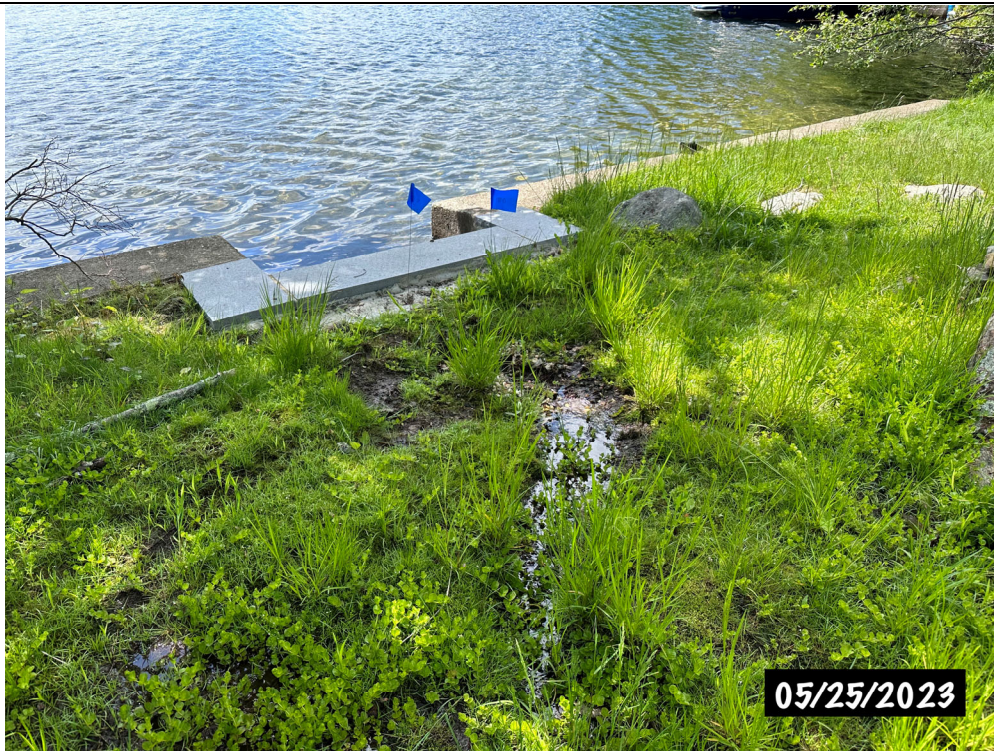
South end of the B-series wetland line near the recently repaired stairs. Notice water flowing toward the steps, which originates from wetland sources.
