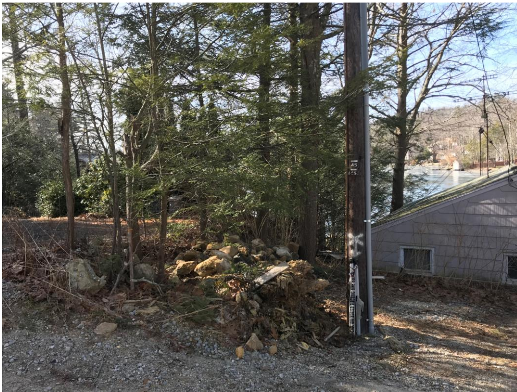
Photo 5: View west of existing pole 45. This existing pole is scheduled for replacement.
