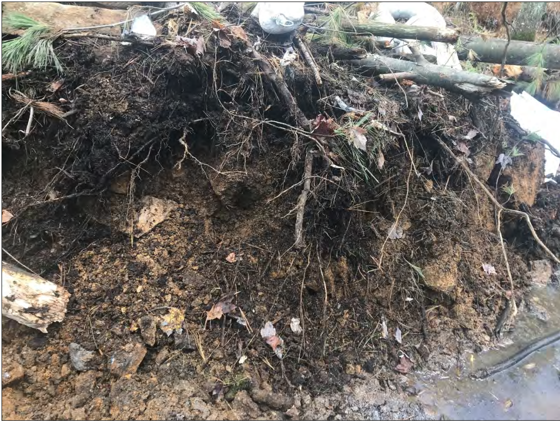
Photograph 38: View of excavation sidewall, looking west. Note coarse fill material present below surface. (10/23/2019)
