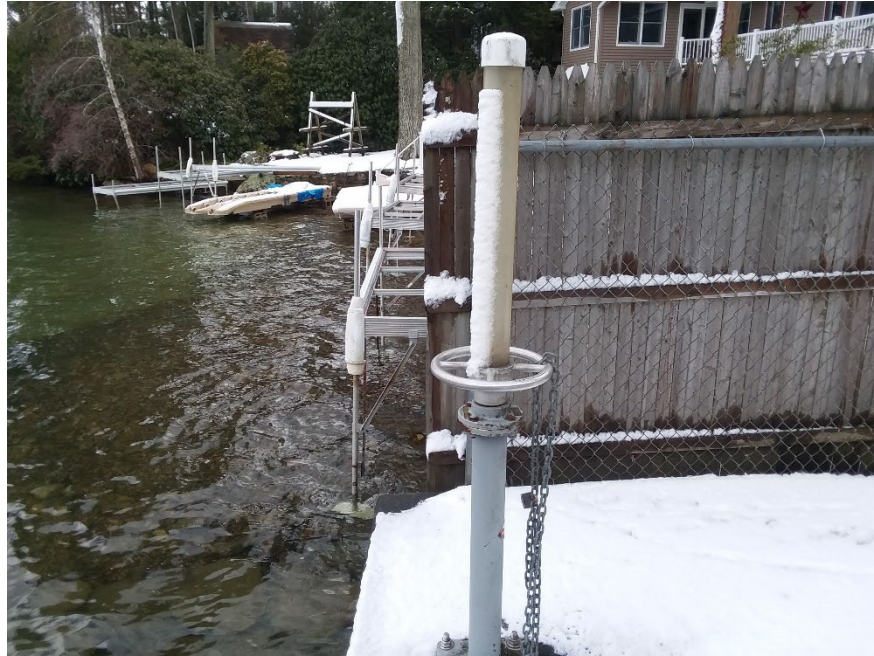
Photo 3: The threaded rod assembly used to raise and lower the plate inside the dam to let water out.
