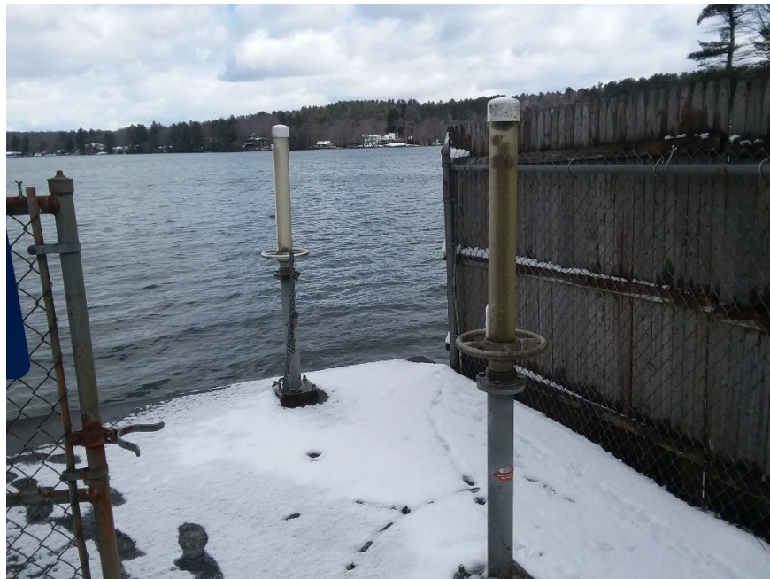
Photo 2: The threaded rod assembly used to raise and lower the plate inside the dam to let water out.
