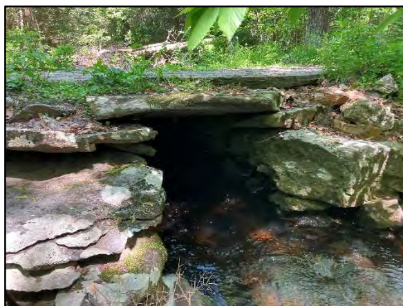
Photo 12. View of the culvert outlet, which is clear of debris, at the Stream S4 trail crossing. Photograph taken May 26, 2022.
