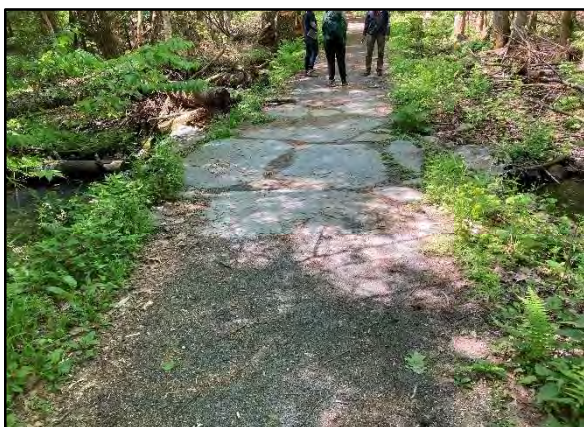
Photo 9. View facing southwest at the Stream S4 trail crossing. No improvements are proposed to the crossing; however, debris has accumulated in the culvert inlet. Photograph taken May 26, 2022.
