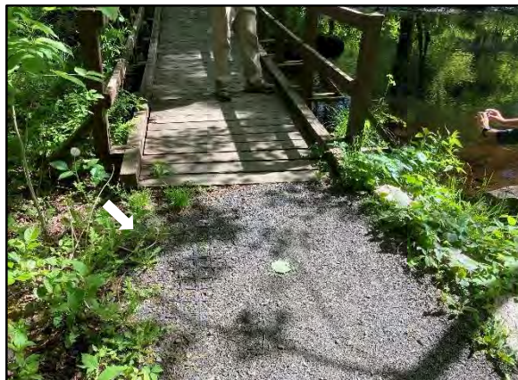
Photo 2. This footbridge is not proposed to be replaced at this time; however, the geogrid beneath the stone dust has become exposed and new stone is proposed to be added to maintain an even trail. Photograph taken May 26, 2022.
