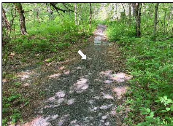
Photo 3. Several sections of trail exhibit exposed geogrid where the top-dressing has worn thin and new crushed stone is proposed to be applied. Photograph taken May 26, 2022.
