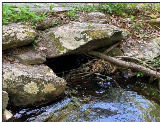
Photo 10. View of the culvert inlet at Stream S4, which has become clogged with organic debris. Photograph taken May 26, 2022.
