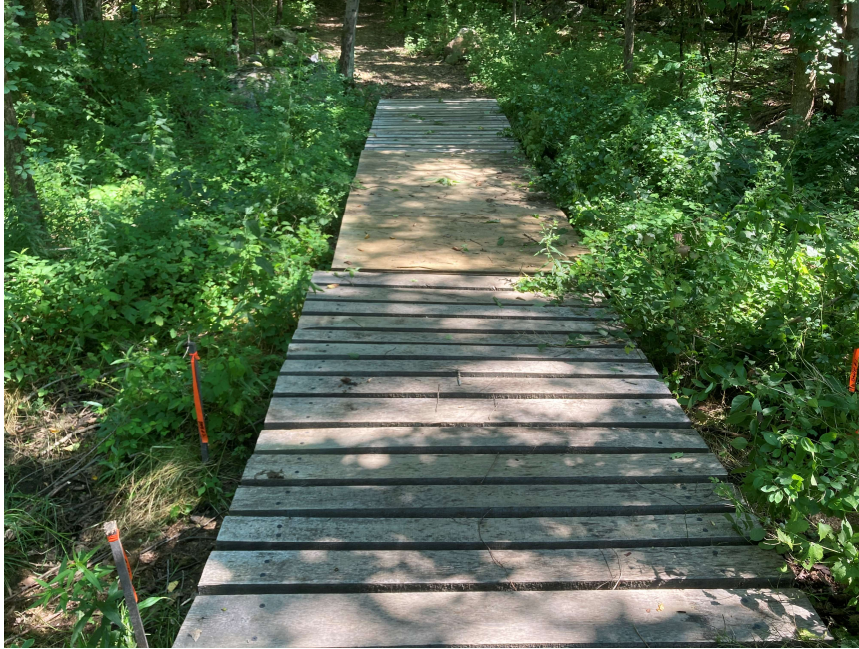
Photo 1 taken by EBT, Inc. on 7/19/2020 – Showing the 40.36’ long foot bridge with a section of plywood decking which needs to be replaced.
