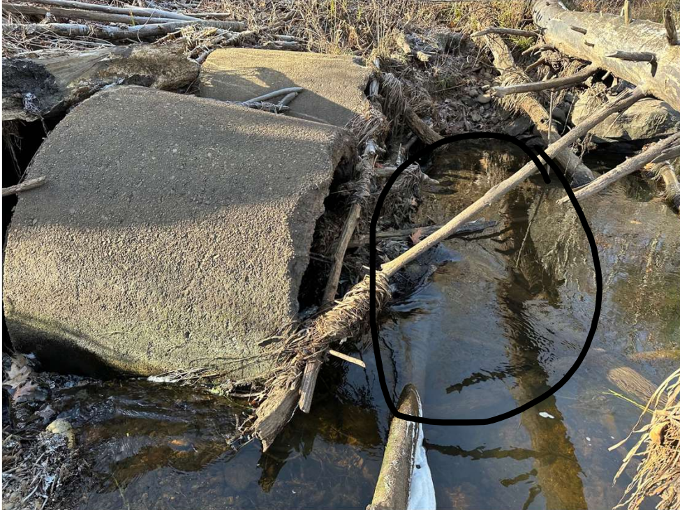
Debris blocking culverts
