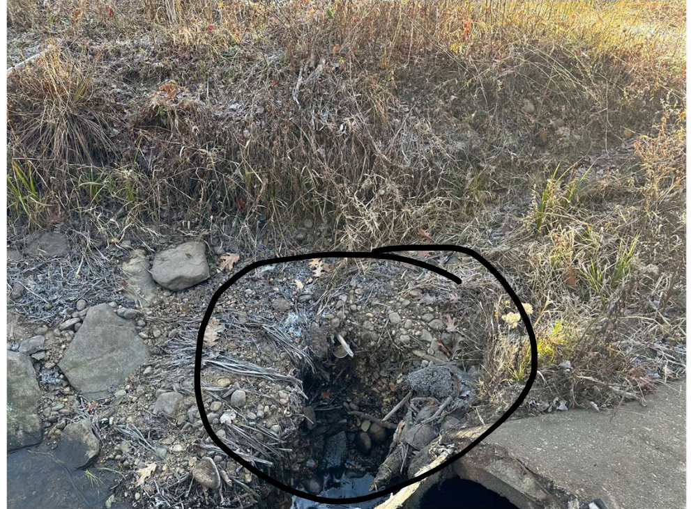
Erosion around culvert opening
