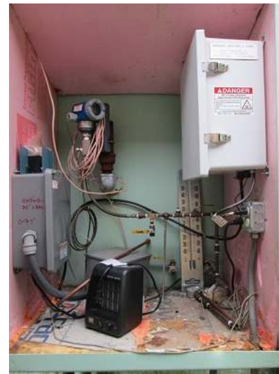
Storage Tank Control Panel (Photo No. 4444)
