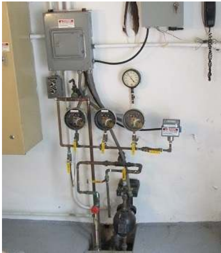
Pumphouse Lower Level - Booster Pump Controls/Gauges (Photo No. 4475)
