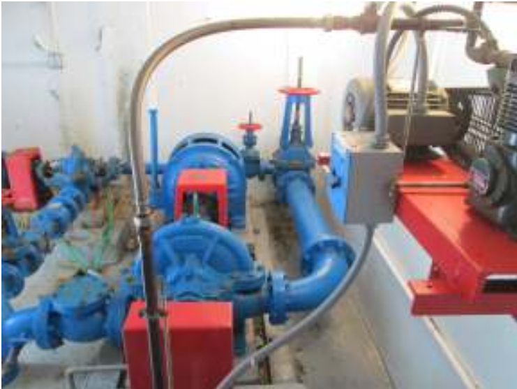
Pumphouse Lower Level – Booster Pumps (Photo No. 4492)
