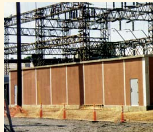
Electrical Substation, Board of Public Utilities
