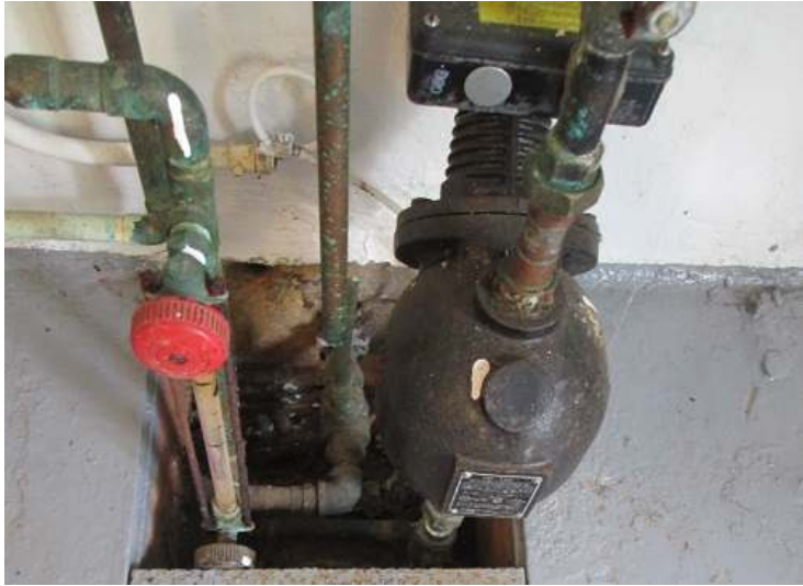
Pumphouse Lower Level – Low Level Cutoff (Photo No. 4477)
