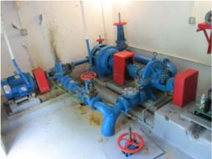
Pumphouse Lower Level – Booster Pumps (Photo No. 4502)
