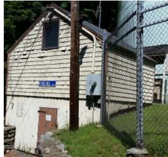
14' x 10' Pumphouse (Photo No. 132127)
