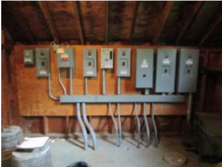
Pumphouse Upper Level – Electrical Components (Photo No. 4453)
