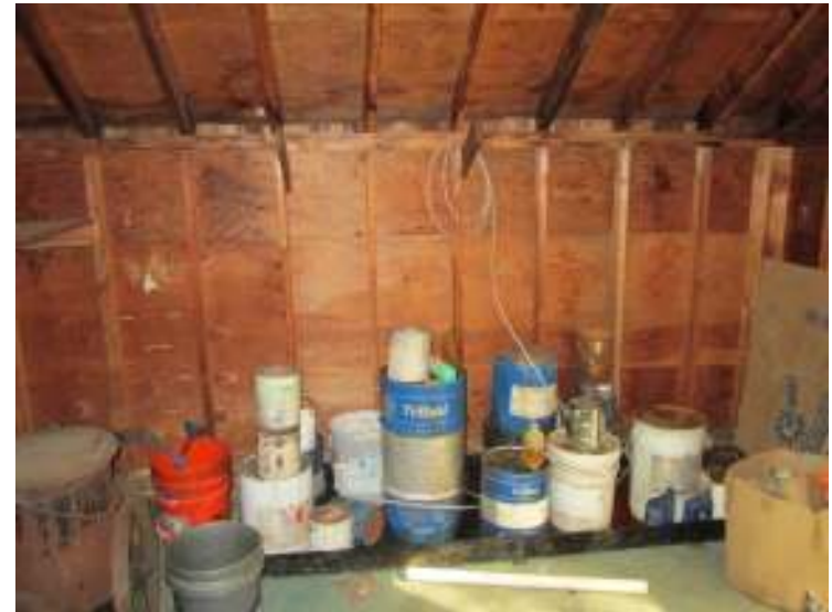
Pumphouse Upper Level – Chemical Storage Area (Photo No. 4454)
