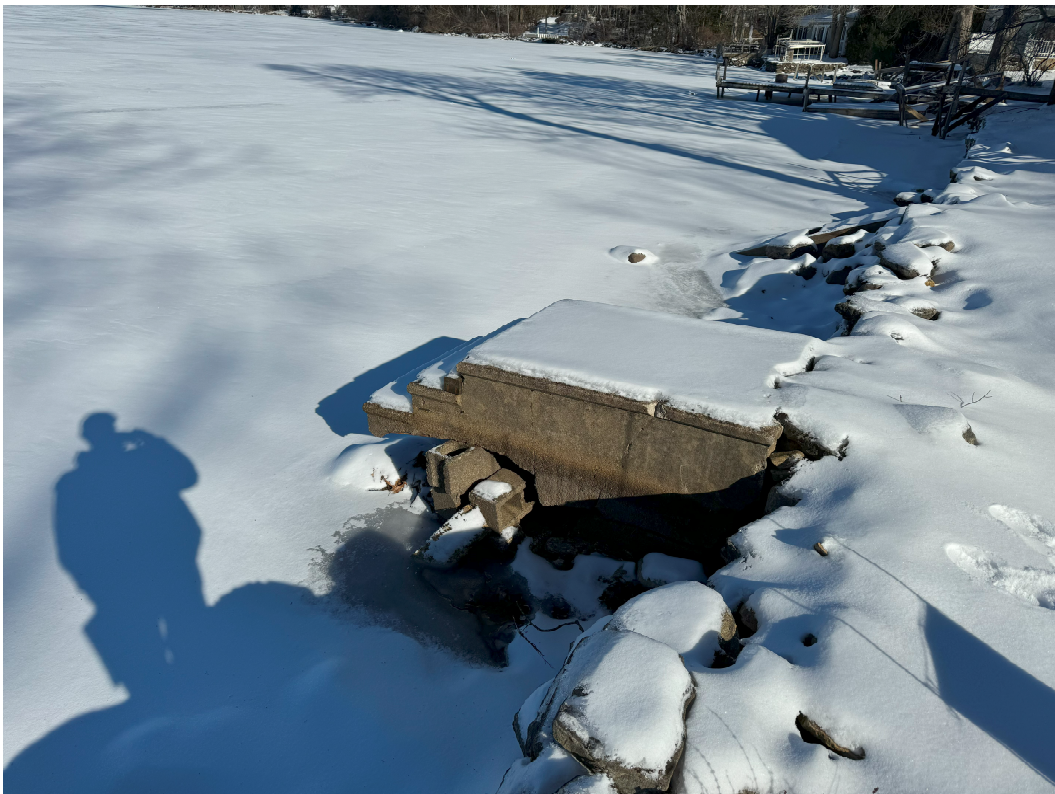
Photo 2 taken by EBT, Inc. on 1/21/2024 – Showing the 30 square foot concrete steps the applicant is proposing to remove abutting the shoreline retaining wall.
