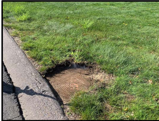
24. Old Farm Road Easement - Manhole ID 635 - Vented manhole cover
