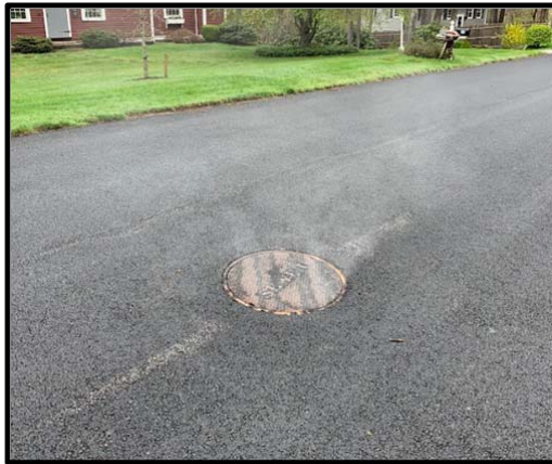
20. Hawthorne Road - Manhole ID 377 - Vented manhole cover
