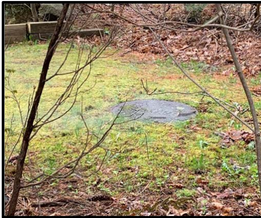
21. Hawthorne Road - Manhole ID 378 - Vented manhole cover
