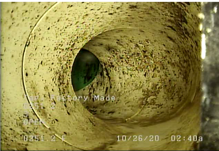
TF - Tap, Factory Made @ 251.2 ft. OPEN
