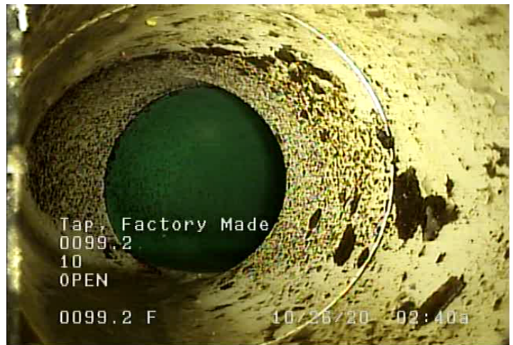
TF - Tap, Factory Made @ 99.2 ft. OPEN
