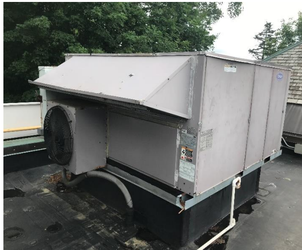
Typical Rooftop Unit
