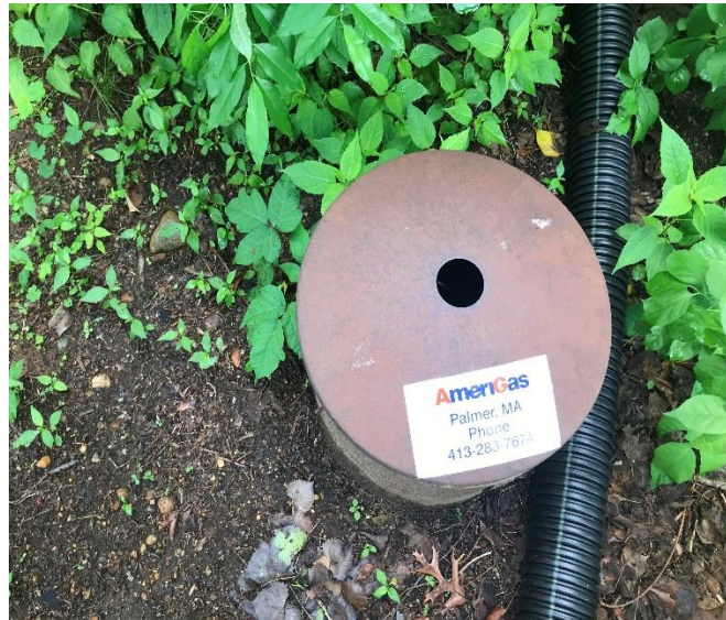
Top of Propane Tank
