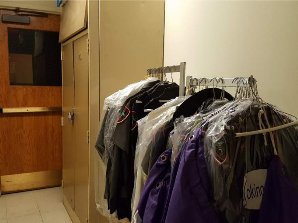
Figure 20: Lack of storage space has led to code violations where egress corridors are blocked by objects within the egress path.
