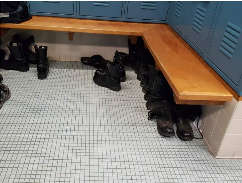
Figure 18: Toilet rooms and locker room facilities are extremely limited and small without adequate or ADA accessible facilities.
