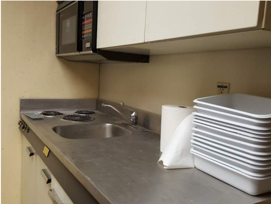
Figure 26: The small unit kitchen is rarely used but should be kept updated for future use by the EOC.
