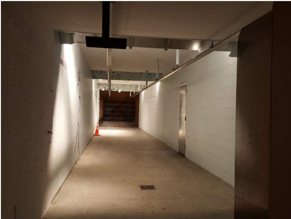
Figure 20: The Firing Range on the Intermediate Level is utilized but the working condition of the exhaust system remains an ongoing issue.
