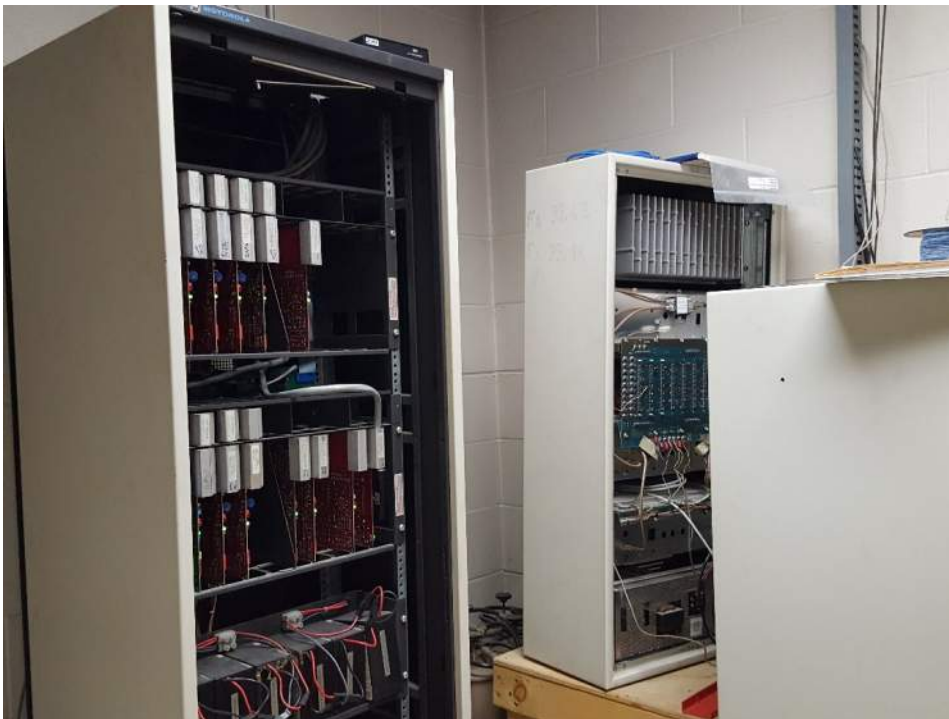
Figure 27: The Radio Equipment Room is an active space that could be better organized and obsolete equipment removed.
