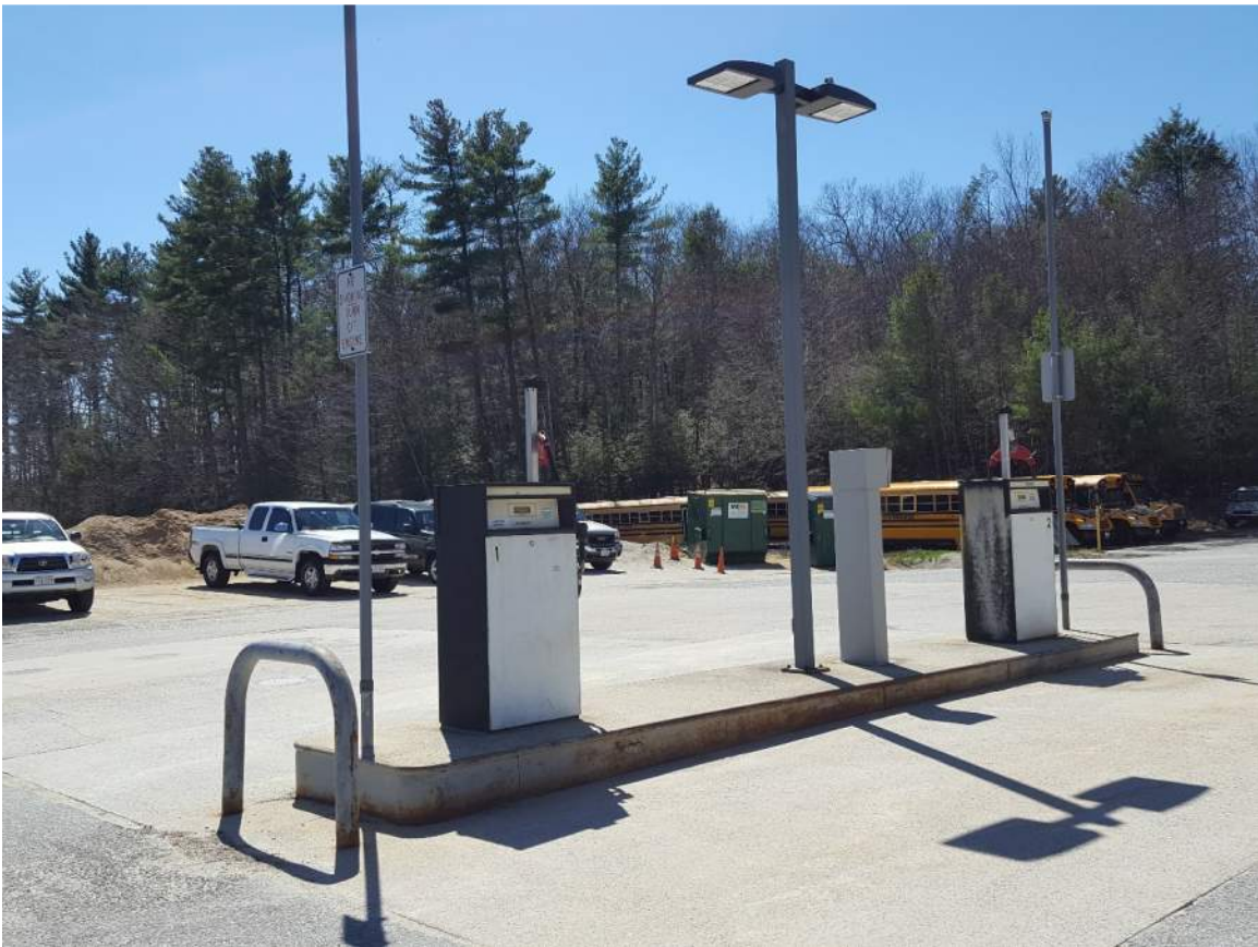
Figure 7: The existing fueling island is in good repair although dispensers will need to be replaced.
