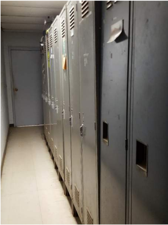
Figure 13: The width of the main Corridor in the Administrative area is impeded by lockers creating building code and ADA compliance issues.
